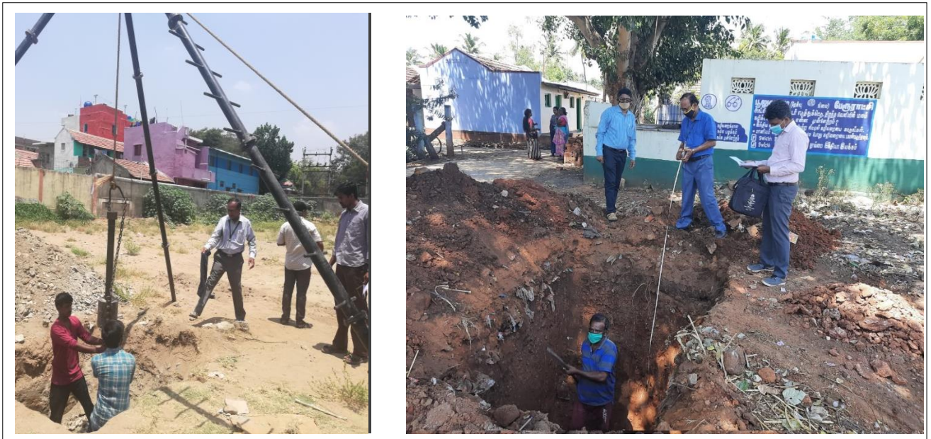
Site investigation and Soil exploration works as part of the Consultancy works carried out through the “Centre for Geotechnical Facility and Services”
