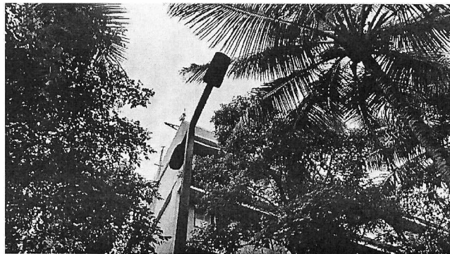
Figure 2: led street lights of -15300w installed and flood lights of 4500w installed
